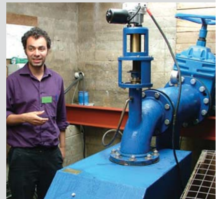
Nick Bard of RD Energy Solutions in the power house at Slochd Mor
